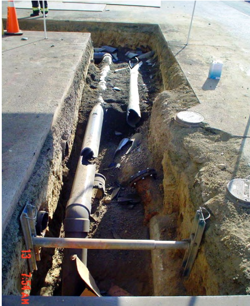
Figure 3-2. Hole in PVC pipe following the explosion
