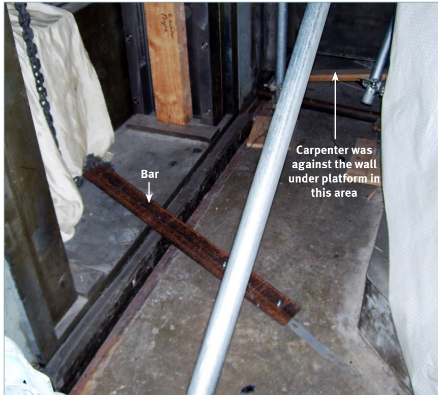
Figure 1-2. Location of bar after falling and area where carpenter was standing
