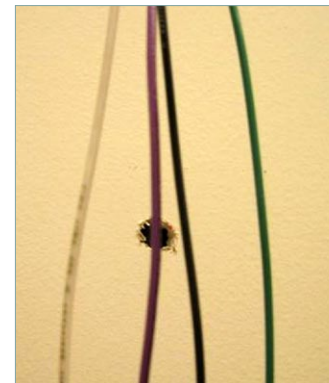
Figure 2-1. Wall penetration and wires pulled from conduit post-event
