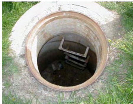
Figure 1-3. Landfill manhole where fatality occurred
