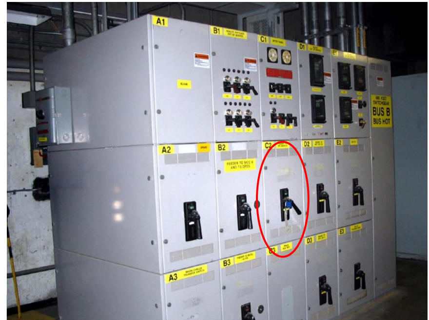
Figure 2-1. Motor Control Center with the 480-volt circuit breaker (circled in red)
