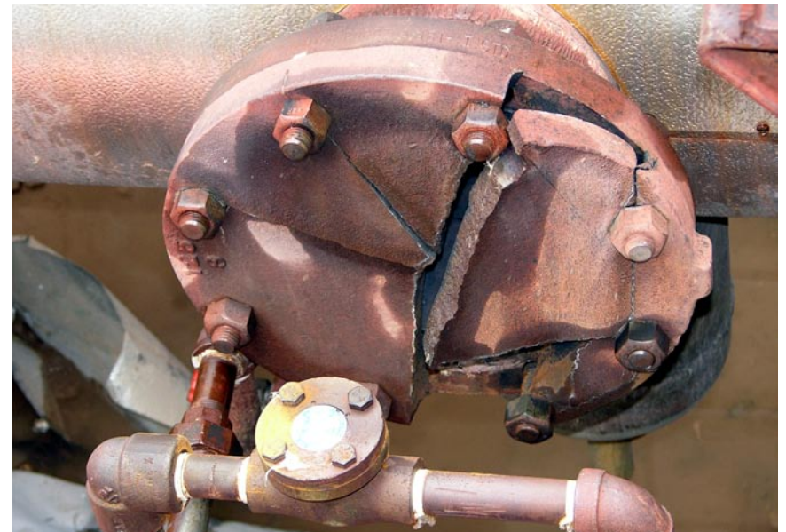
Figure 1-1. Failed blind flange
