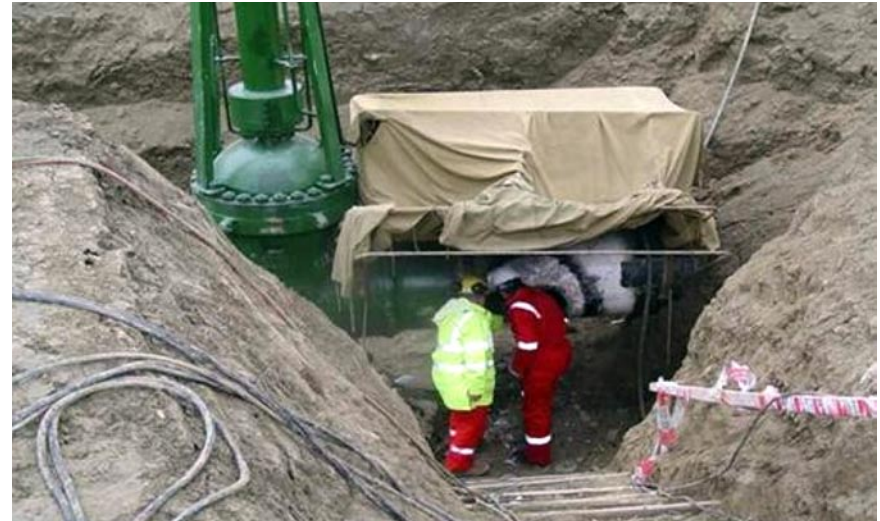
Figure 1-1. Gate valve (green) and pipe section under tarp where fire occurred
