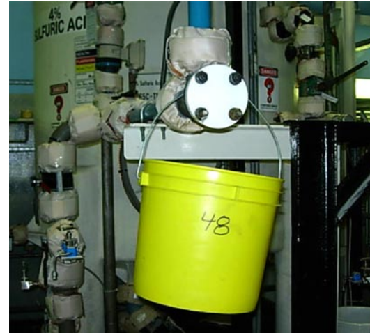
Figure 3-1. Blind flange with catch bucket
