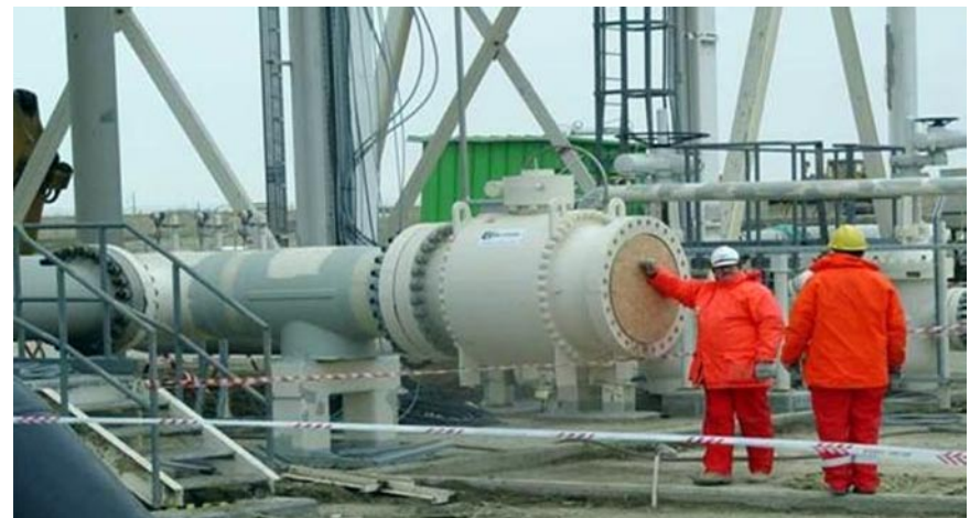
Figure 1-2. The ball valve and point of entry into the 30-inch pipeline
