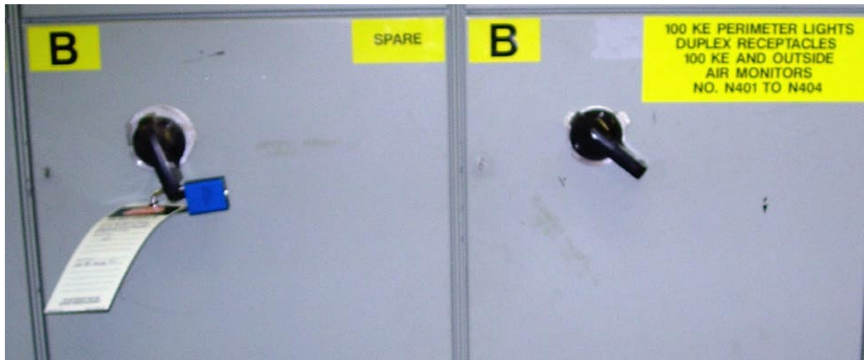
Figure 1-1. Side-by-side circuit breakers showing the lock and tag on the SPARE
