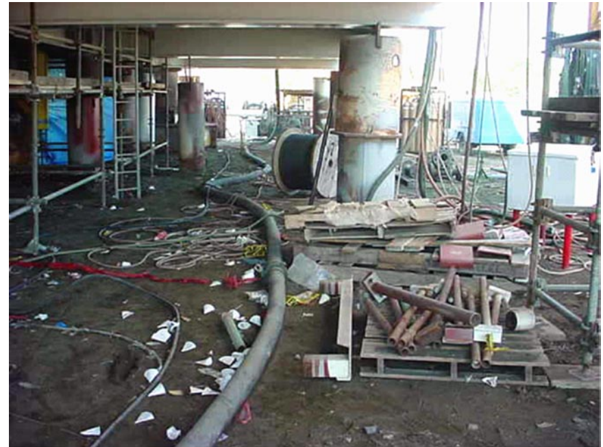
Figure 3-2. Can you find the tripping hazard?
