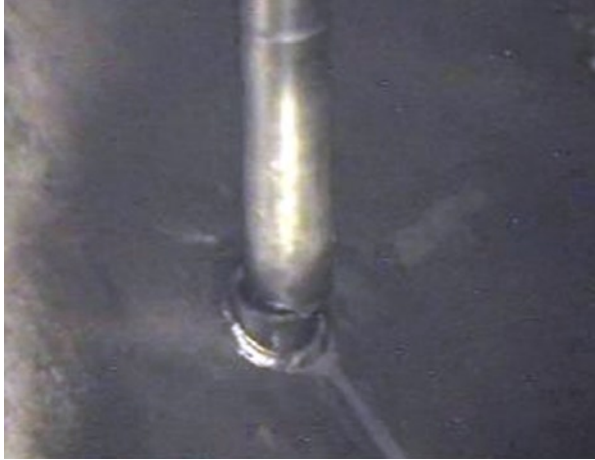
Figure 4-2. Failed pipe nozzle on tank head
