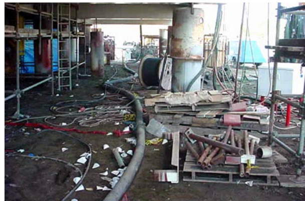
Figure 3-2. Can you find the tripping hazard?
