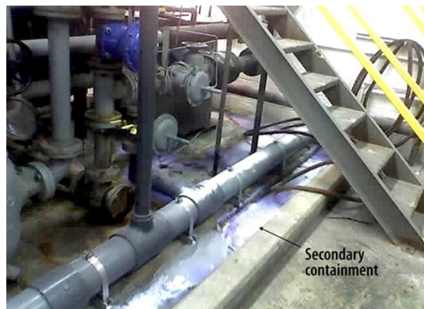
Figure 4-1. Secondary containment with neutralization results
