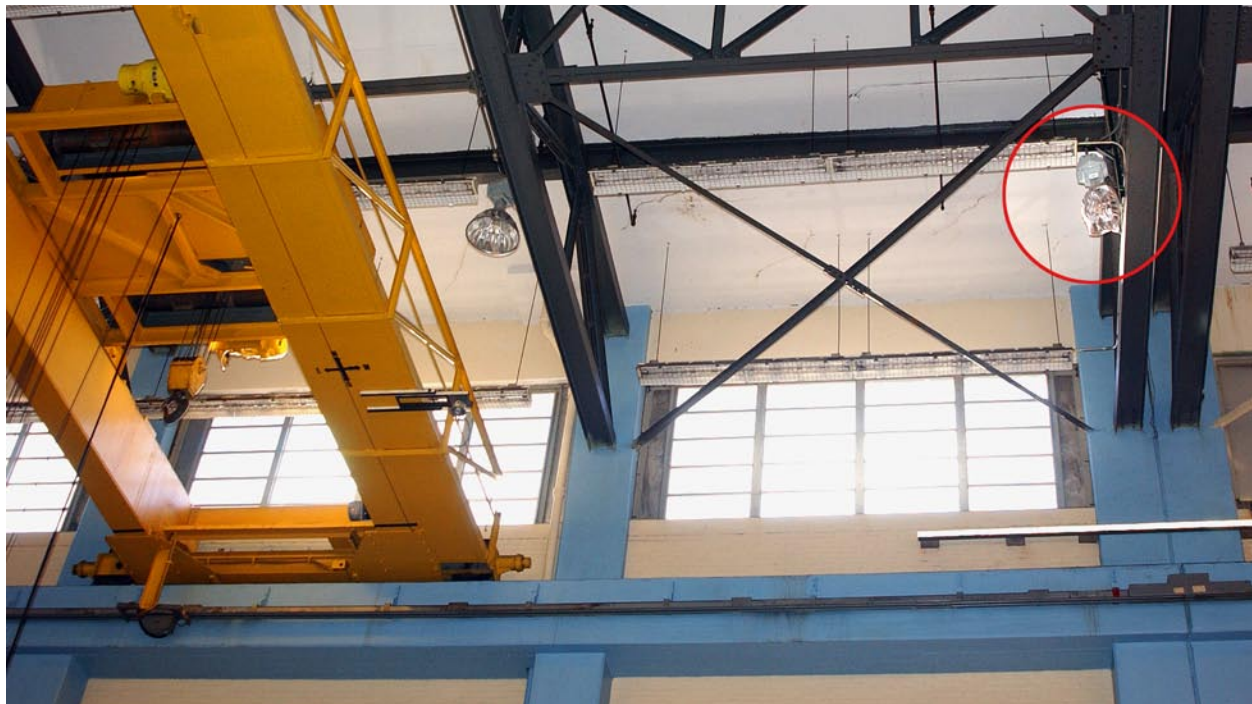
Figure 2-1. Broken light fixture
