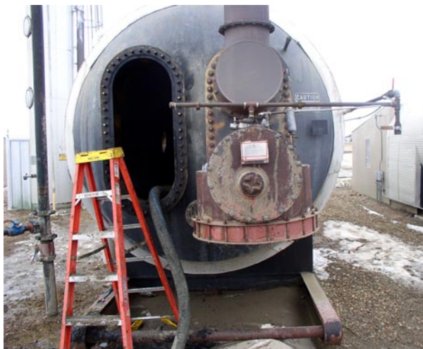
Figure 1-1. Vessel and injured worker's ladder
