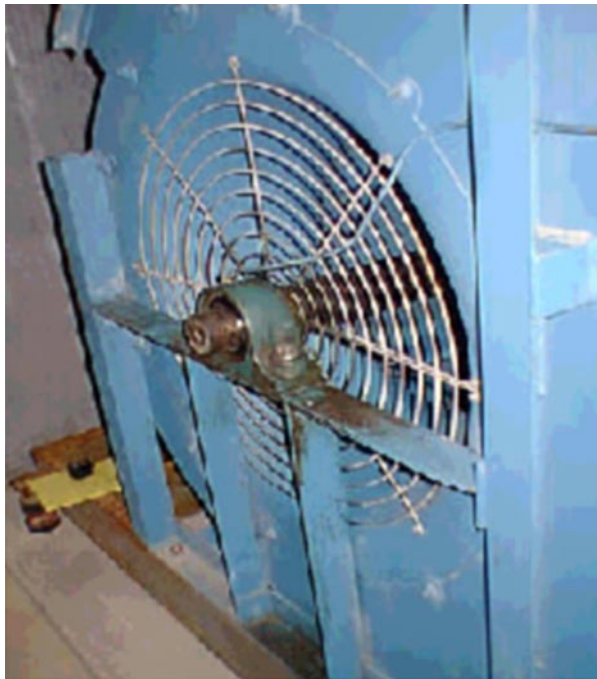
Figure 4-3. Exposed shaft end of the fan unit
