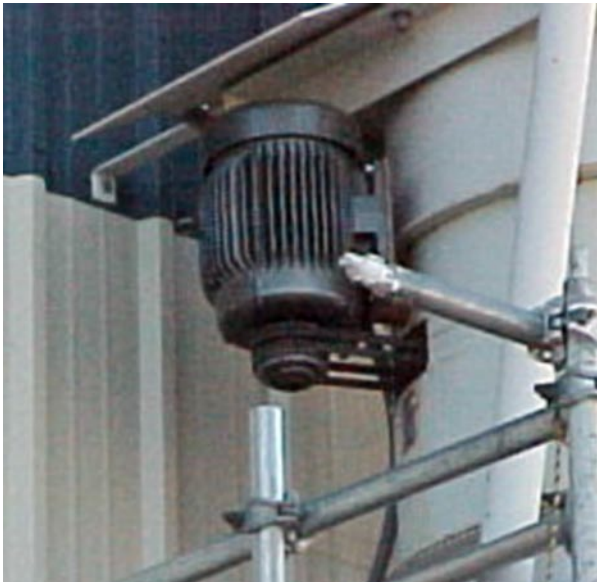
Figure 4-5. Blower motor with unguarded fan belt
