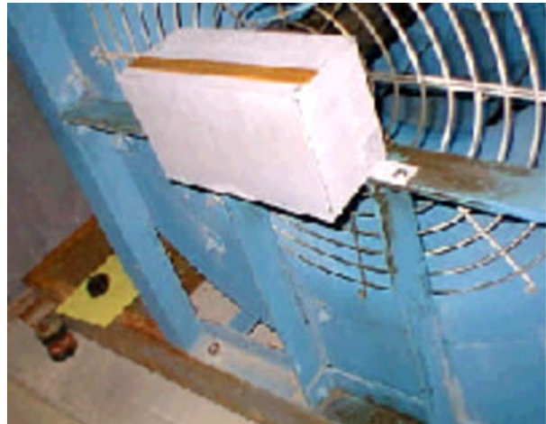
Figure 4-4. Fan with guard installed over shaft end
