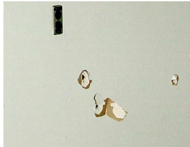
Figure 3-4. Wall penetrated by projectiles
