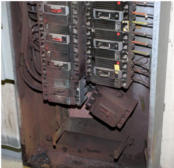
Figure 3-1. Arc-damaged circuit breaker in panel position 12 hanging by the phase C connection
