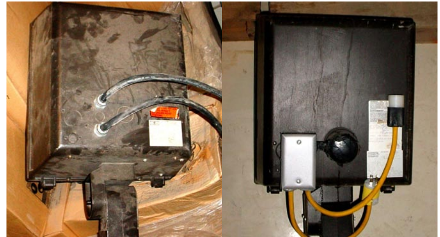
Figure 2-4. Back of previously modified (left) light unit and corrected modification (right)
