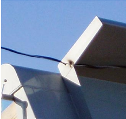
Figure 1-2. Severed power lines held in place by support cable
