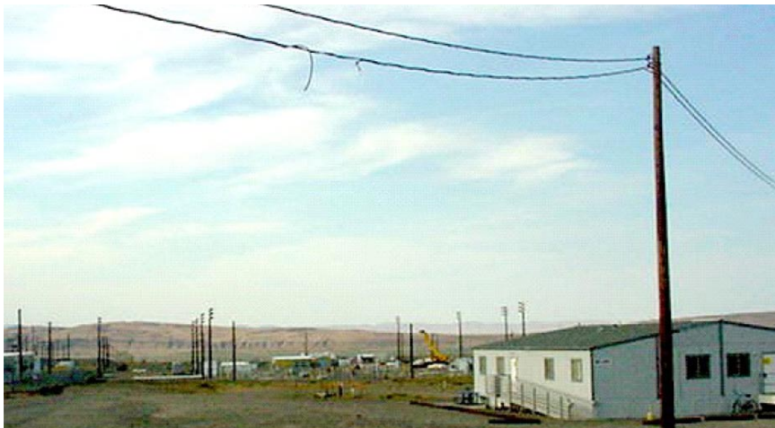
Figure 1-3. Cut power line running diagonally across the road bed
