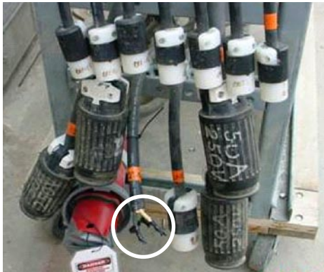
Figure 4-1. Pigtails on the back of the mini load center and the exposed wires that arced (circled)
