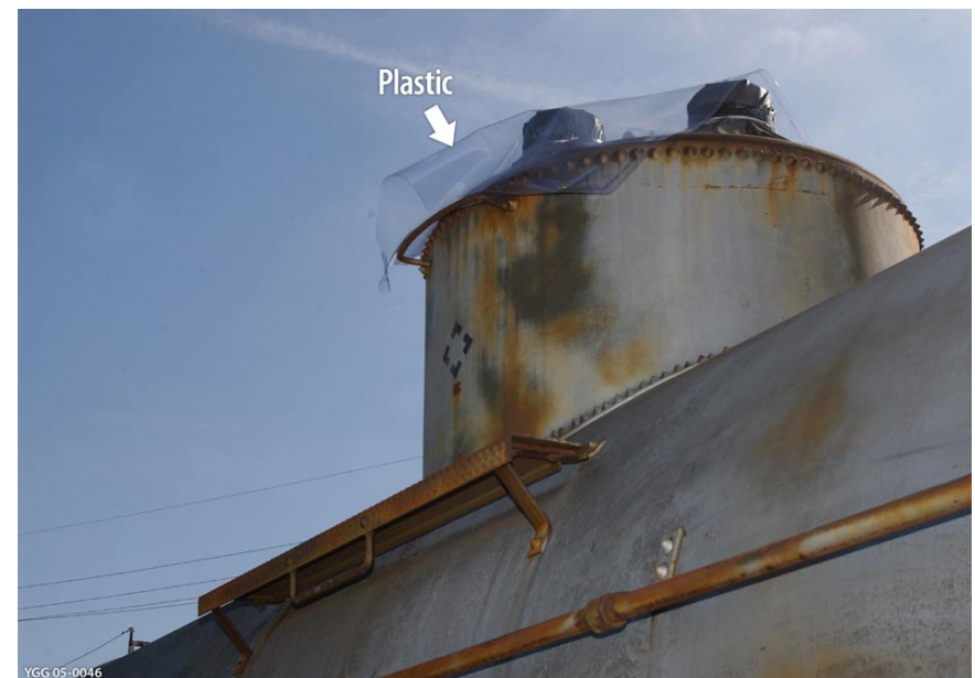
Figure 4-1. Plastic on rail tank car hatch
