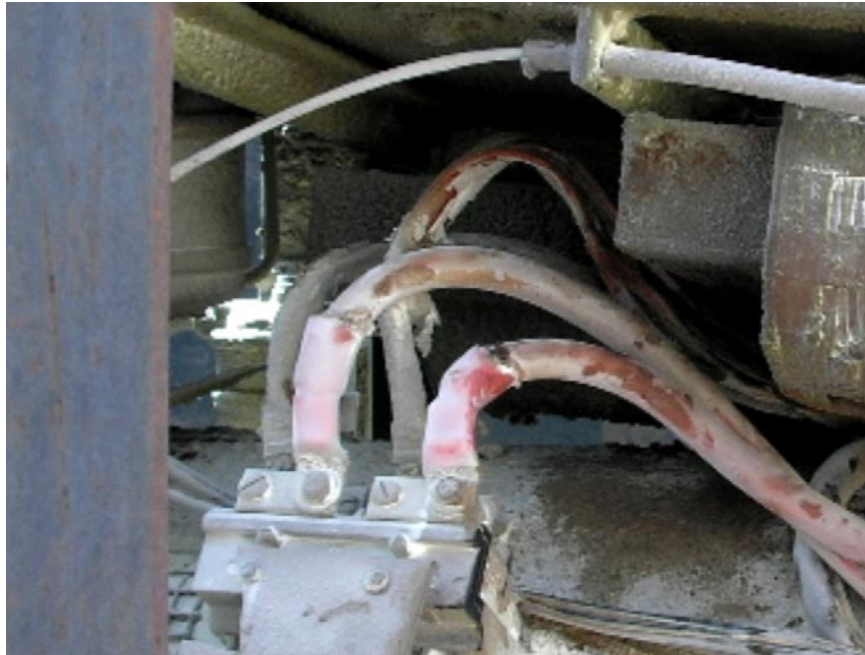
Figure 2-2. Cracked insulation on cables
