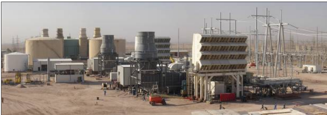
Electric Generation Plant
