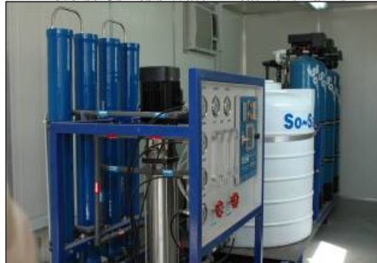
Reverse Osmosis Water Treatment Tanks
