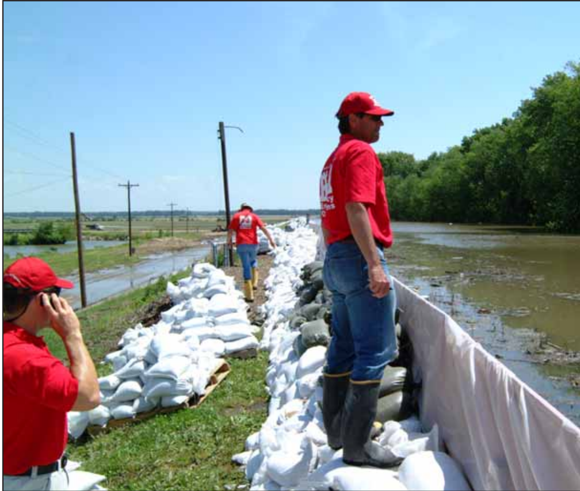
Working alongside a temporary batter board and sandbag floodwall, Terry Jorgensen (center), St. Paul District; Joe Dziuk (left), and Glen Hotchkiss (background), Rock Island District, survey rising waters at the South River Drainage District just north of Hannibal, Mo., during the hot afternoon hours of June 18.
