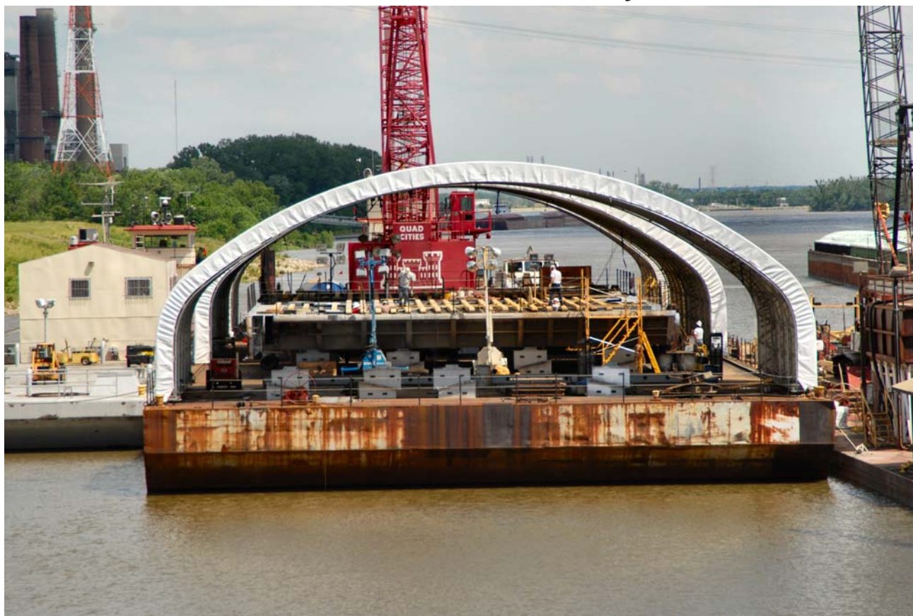
The District's heavy-lift crane, the Quad Cities, can be seen in the background of the barge housing one of the gates for the Melvin Price main lock chamber. The gates were housed on covered work barges, while diagonal braces on the miter gates were replaced, allowing the tension to be adjusted from the top without the necessity of dewatering the lock. Photo by Alan Dooley, Public Affairs, St. Louis District.
