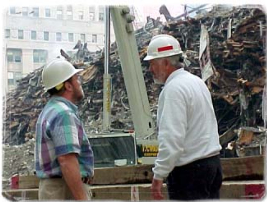
Allen Morse, debris management, Mobile District (right), talks with Ben Turner, president, Phillips and Jordan Construction, Inc. (left), about the details and complications of debris removal at the World Trade Center disaster site in New York City.
