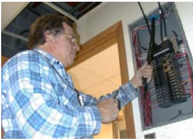
Mike Milobar, Saylorville Maintenance Crew, takes a look at the electrical wires near the kitchen closet. Above in the top left photo, John Greif works moves equipment around the maintenance garage.
