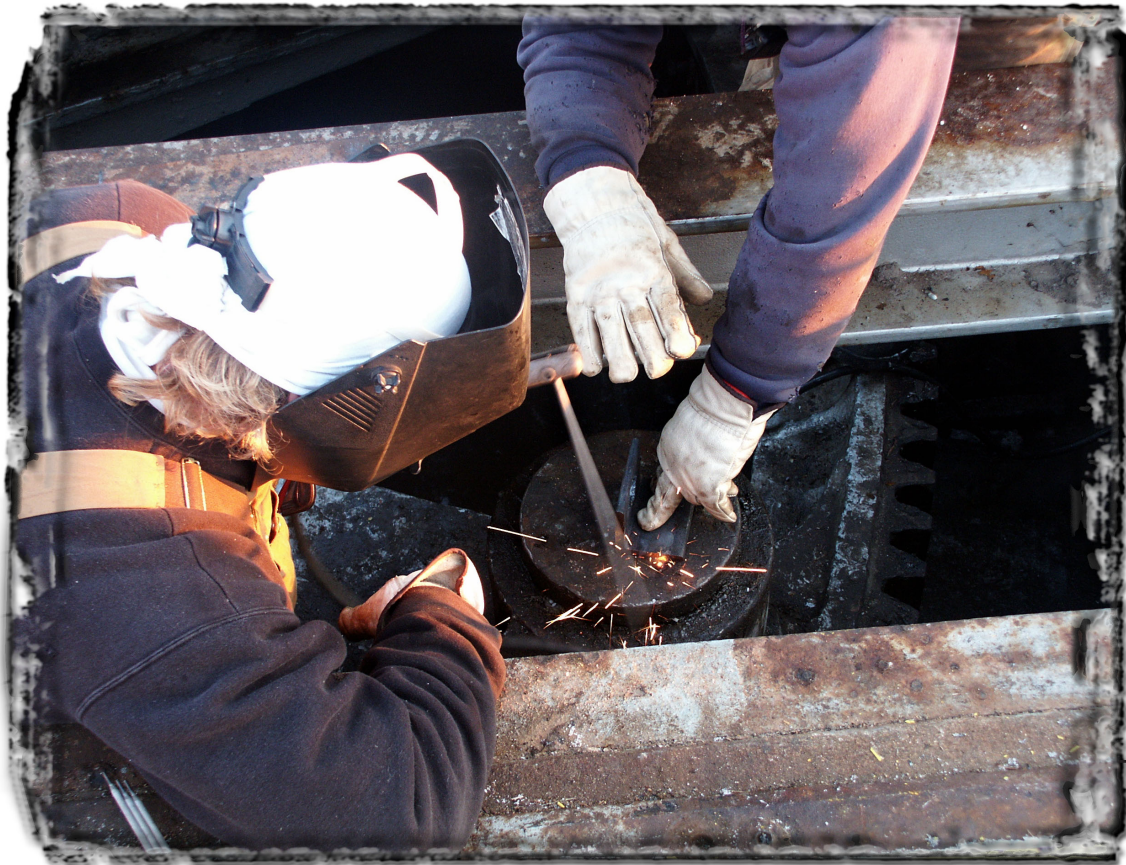
Members of ILWW Maintenance units weld a new strut arm into position as part of the emergency repairs involved in replacing a fractured buffer box at Starved Rock Lock and Dam.
