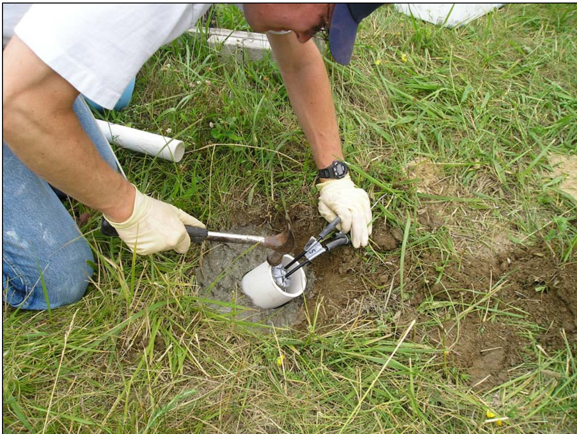
Figure A-5. Tension lysimeter installation.
