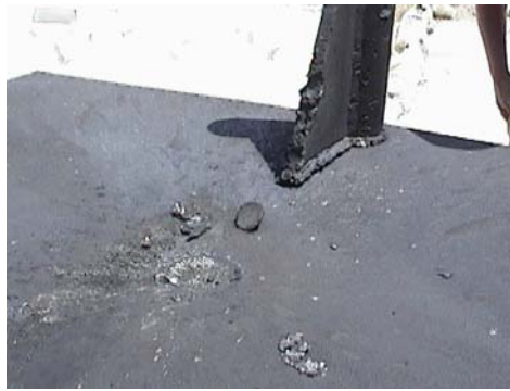
b. Picture shows cracked weld at the shadow pole
