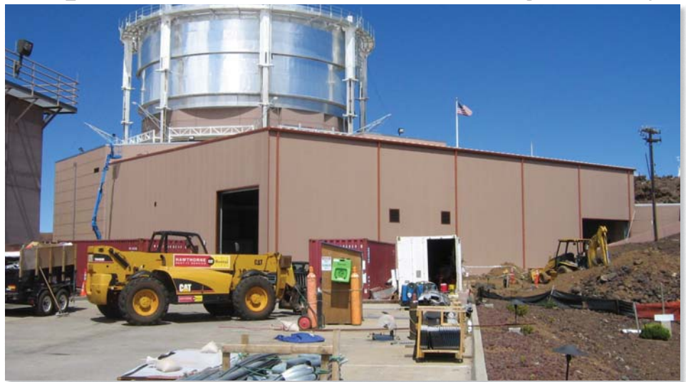
The Mirror Coating Facility (above) as it appeared in August 2007 during construction at the Maui Space Surveillance Complex. Ribbon-cutting ceremonies were held simultaneously last month in the new building and at the Institute for Astronomy, Pukalani, Maui. Courtesy photo
