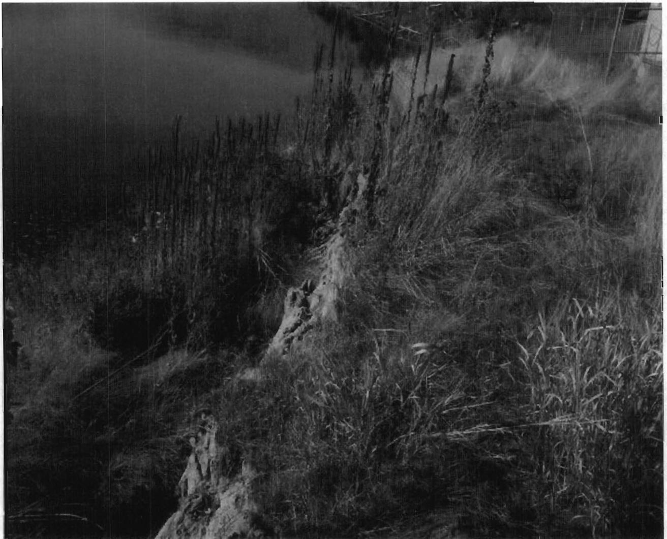
Photograph of project site showing sloughing that occurred after the flood events in June 2006.
