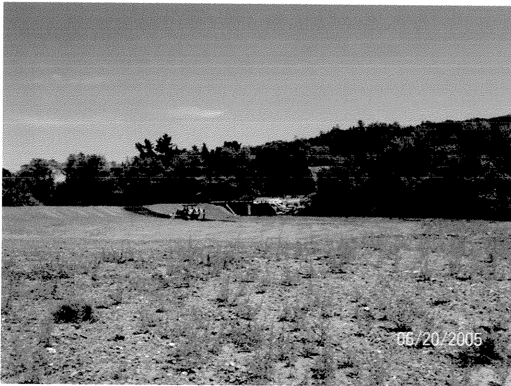
Photo 5. Washington School Road at Asti Russian River Summer Crossing Constructing the Gravel Approach.
