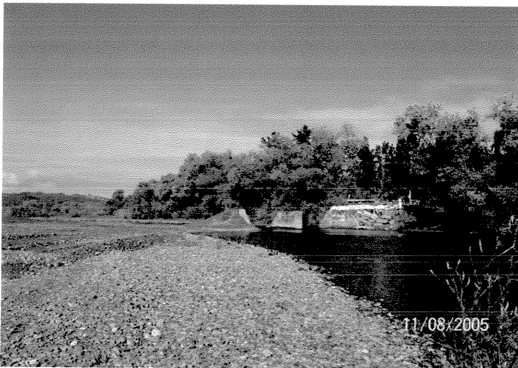
Photo 6. Washington School Road at Asti Russian River Summer Crossing After the Removal of the Deck and Approach Roadway.
