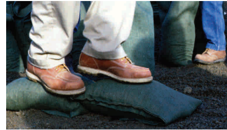
Place each succeeding bag tightly against and partially overlapping the previous one. Compact and shape each bag by walking on it.
