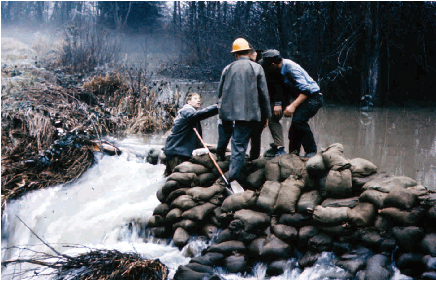
This classic shot shows conditions frequently are not even close to perfect. In the early '50s, flood fighters moved fast and furious to contain the swollen Snohomish River at Ebey island - a major flood event.
