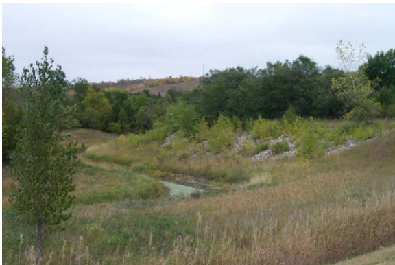
Figure 2.27 MINIMALLY ACCEPTABLE. Trees and saplings are becoming established within riprap-protected areas and along the lower portions of the river channel, and must be removed. (ND)
