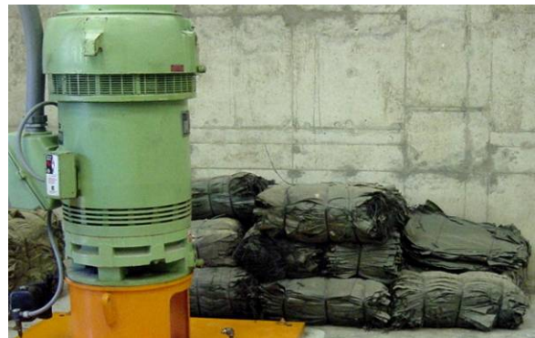
Figure 3.2 Sandbag storage in a levee pumping station. (OK)
