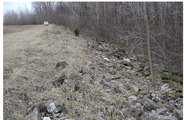
Figure 2.28 UNACCEPTABLE. Tree and sapling growth is well established within the riprap protection on an earthen levee. This overgrowth must be removed. (MO)
