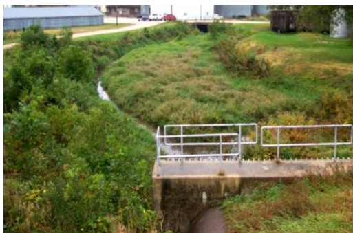
Figure 2.56 UNACCEPTABLE vegetation and sediment in interior drainage channel. (IA)
