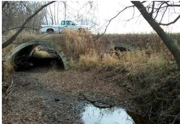
Figure 2.59 The culvert on the left is Minimally Acceptable with sediment accumulation within the culvert. The culvert on the right is totally unacceptable with 2/3 of its flow capacity reduced by sediment and debris. This project was rated as UNACCEPTABLE because of the reduced flow capacity of the culverts. (MN)
