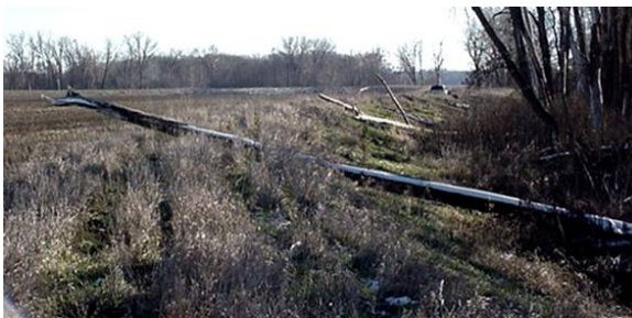
Figure 2.9 UNACCEPTABLE encroachments on earthen levee. Fallen woody debris requires removal. (KS)
