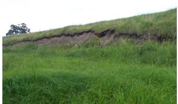
Figure 2.17 UNACCEPTABLE earthen embankment failure. (MN)
