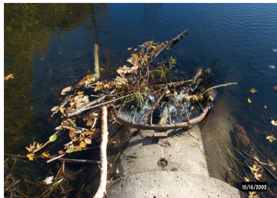
Figure 2.22 Beavers attempting to block the culvert passing through a gated embankment. (MN)
