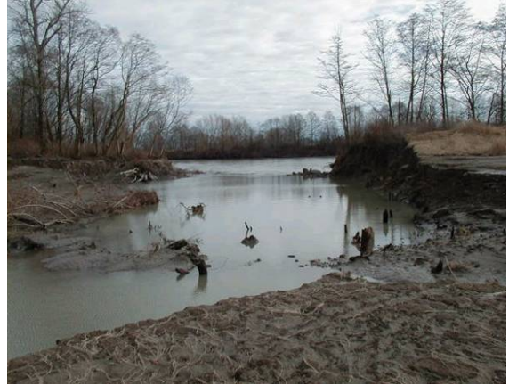
Figure 6.1, Levee breach in Lynden, WA (NWS)
