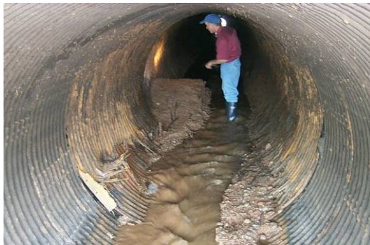
Figure 2.61 UNACCEPTABLE, Failing corrugated metal pipe. DO NOT WALK INTO A FAILING CULVERT LIKE THIS. This section has actually separated, allowing the surrounding soil to enter the pipe and the overburden to collapse. This sponsor was denied rehabilitation assistance due to this maintenance deficiency.
