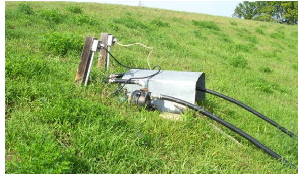
Figure 2.8 UNACCEPTABLE encroachment. Piping for lawn irrigation system drilled through levee without approval. (ND)
