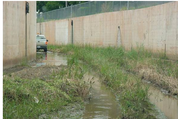
Figure 2.75 UNACCEPTABLE vegetation and extensive sediment in channel. (TX)
