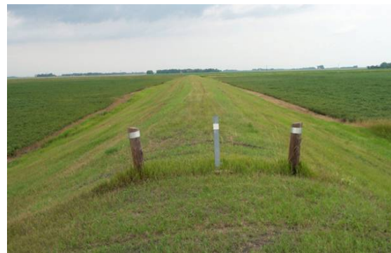
Figure 2.5 MINIMALLY ACCEPTABLE. Field encroaches on levee easement. The landowner has tilled the soil right to toe of the levee, and was requested to stay back at least 10 feet. (ND)
