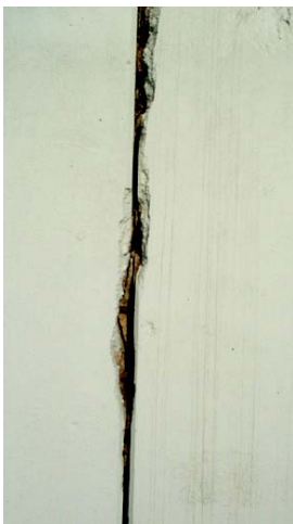
Figure 2.45 UNACCEPTABLE exposed rebar. Monolith joint separation with exterior spalling along the joint and interior spalling in the area of the rebar. (MN)
