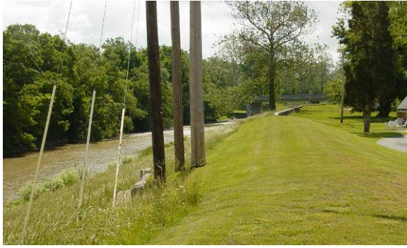
Figure 2.7 UNACCEPTABLE levee encroachments. Utility poles in levee embankment. (IN)
