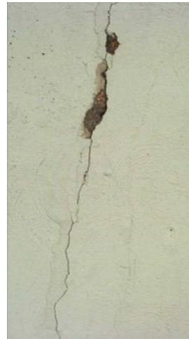
Figure 2.44 MINIMALLY ACCEPTABLE Vertical floodwall crack with spalling. The rating for this particular crack is Minimally Acceptable because the crack is still tight but there is some spalling occurring as well. (MN)
