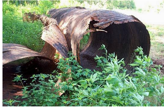
Figure 2.62 Pieces of the same pipe, once removed from the levee. Note that while much of the pipe may have appeared to be in good condition from the inside, the outside was extremely corroded. The public sponsor attempted to patch the pipe the first year, but when it failed again, the entire CMP was replaced.
