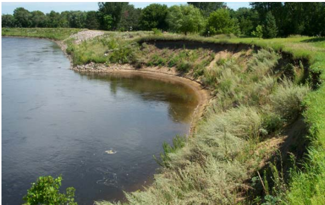
Figure 2.24 Channel erosion located at the upstream end of a flood control levee protected by riprap. Erosion caused by riprap protection and eddy currents. (MN)
