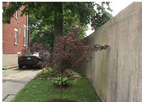
Figure 2.52 UNACCEPTABLE. Trees growing too close to floodwall. (KY)
