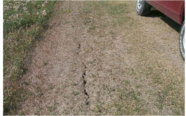
Figure 2.33 ACCEPTABLE cracking in clay levee with shrinkage cracking caused by dry conditions. (MN)
