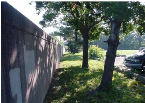
Figure 2.51 UNACCEPTABLE. Trees growing too close to floodwall. (KY)
