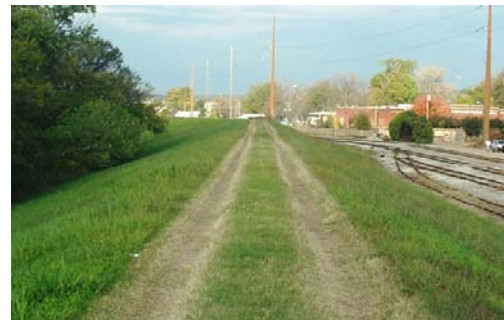
Figure 2.39 UNACCEPTABLE rutting in levee. (OK)
