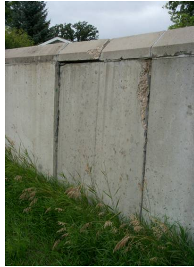
Figure 2.49 UNACCEPTABLE monolith movement in floodwall. The monolith shown in the photo has tilted about 6 inches riverward as well a vertically. Note the movement when compared to the adjoining monolith and the top cap. As the monolith moved considerable spalling has occurred along the joint. This project is monitored very closely during flood events. (ND)
