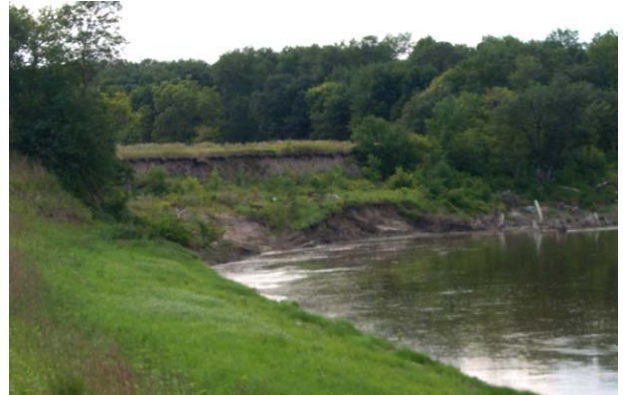
Figure 2.16 UNACCEPTABLE. Slope failure and erosion on a channel improvement project. (MN)
