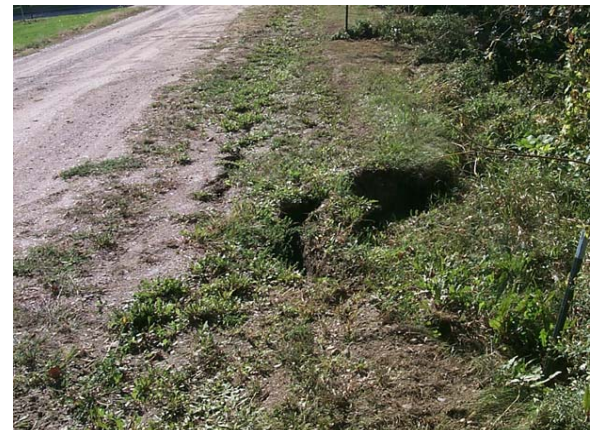
Figure 2.35 UNACCEPTABLE embankment cracking and slope failure. This photo shows what started out as cracking along the crest of the embankment and quickly developed into a slope failure. All cracking located on a levee or riverbank must be closely monitored. (MN)
