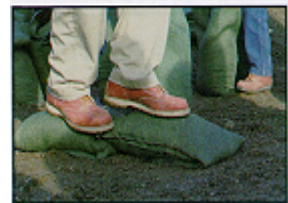
Place each succeeding bag tightly against and partially overlapping the previous one. Compact and shape each bag by walking on it.
