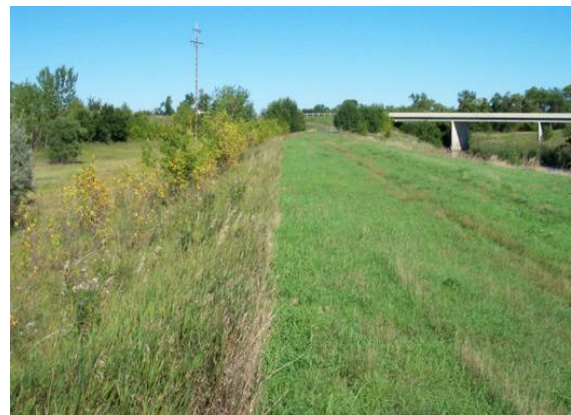
Figure 2.32 UNACCEPTABLE long grasses and trees on levee side slopes. (ND)
