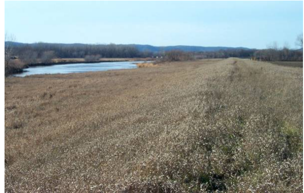
Figure 2.30 UNACCEPTABLE levee with knee-high grass, making visual inspection nearly impossible. (MN)
