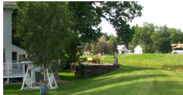
Figure 2.14 UNACCEPTABLE encroachment. Patio construction using railway timbers and fill without approval. (ND)
