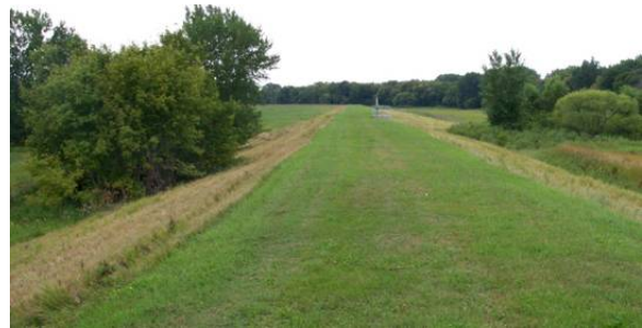
Figure 2.31 UNACCEPTABLE. Levee is mowed but trees and longer grasses within levee easement area. Trees are greater than 2” in diameter. (MN)
