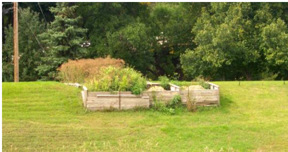
Figure 2.13 UNACCEPTABLE encroachment. Gardens and compost bins located on levee crest and riverward slope. (ND)
