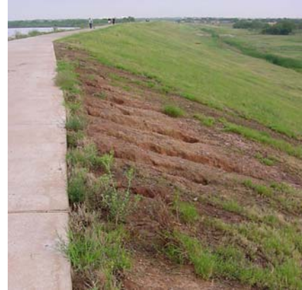
Figure 2.1 UNACCEPTABLE erosion of levee slope. (TX)
