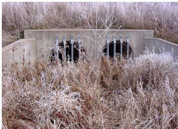
Figure 2.60 MINIMALLY ACCEPTABLE, vegetation blocking the concrete culvert must be removed. (KS)
