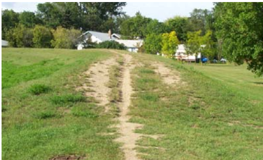
Figure 2.36 MINIMALLY ACCEPTABLE levee rutting caused by pedestrian and bicycle traffic. (ND)
