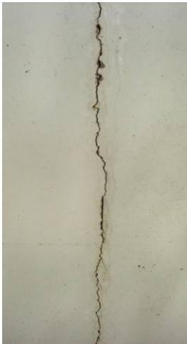
Figure 2.43 MINIMALLY ACCEPTABLE 1/8 th inch crack extends through concrete floodwall and needs to be sealed to prevent further damage. (MN)
