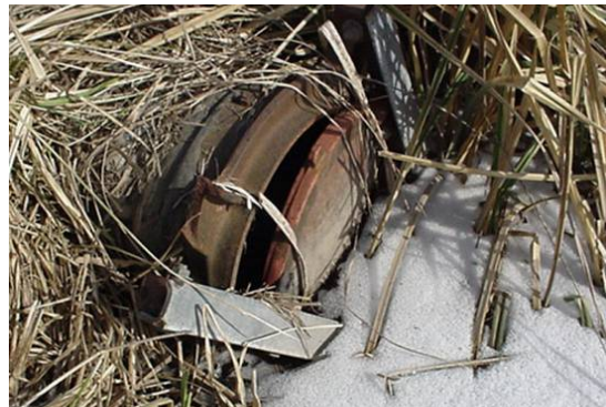
Figure 2.66 UNACCEPTABLE flap gate in earthen levee. (Broken hinge and vegetation growth.) (MO)
