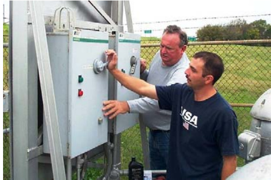
Figure 7.1, Inspection of pumping station controls. (OK)
