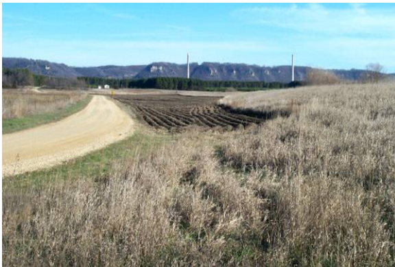
Figure 2.6 UNACCEPTABLE levee encroachments. This landowner tilled near one third of the way up the landward levee slope. (MN)
