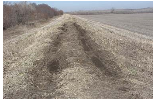
Figure 2.37 UNACCEPTABLE ruts in levee crown require fill. (MO)
