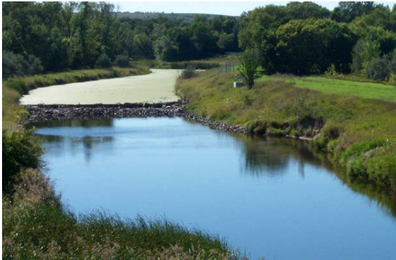
Figure 2.15 UNACCEPTABLE. Slope failure and erosion caused by inadequate channel bottom and side slope protection. This was a direct result of bottom scouring that undercut the levee slope and erosion caused by turbulent flow at the end of the bank protection. (ND)
