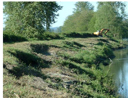
Figure 2.3 Slope failure on bank protection project. (WA)
