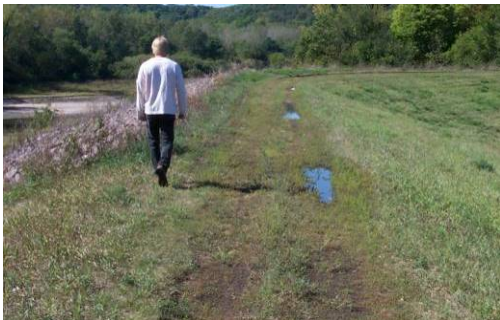
Figure 2.38 MINIMALLY ACCEPTABLE ponded water along a levee crest. (MN)
