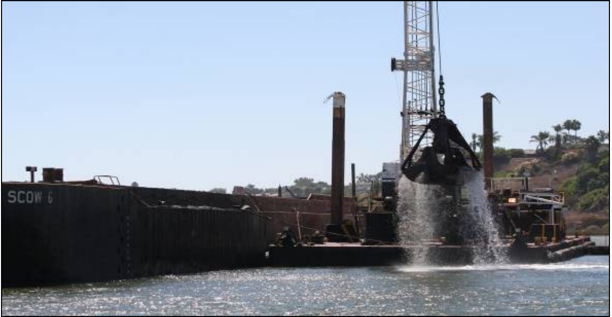
Clamshell Dredge with 5 cubic yard bucket and 3000 cubic yard scow, dredging Sediment Basin II.
