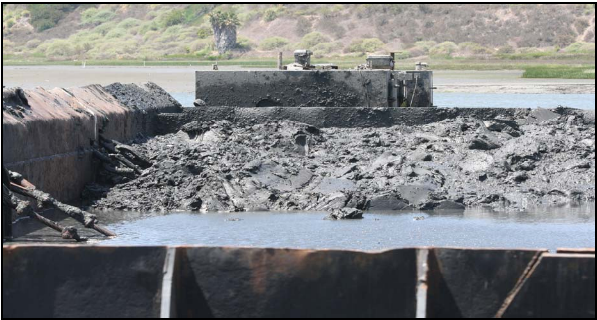
View inside scow being loaded with sediment for disposal at LA-3, 8 June 2007
