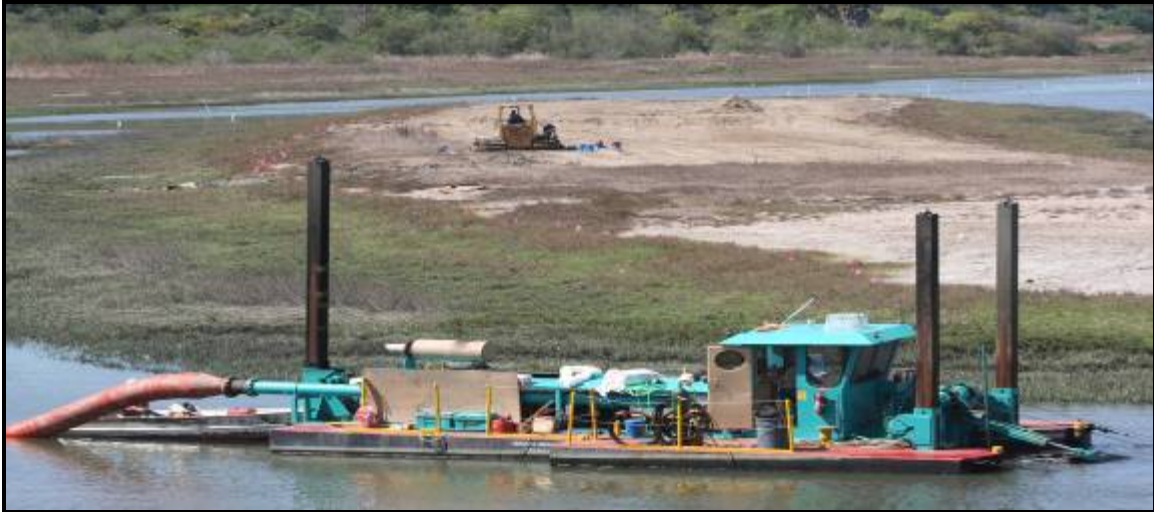
Dredging Hotdog Tern Island Restoration Channel and resurfacing Hotdog Island, Photo by Keane Biological, March 2007
