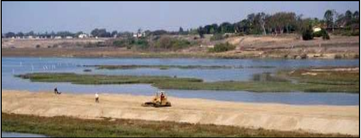
Hotdog Island with beginning of sand capping, Photo by Keane Biological, 3 April 2007
