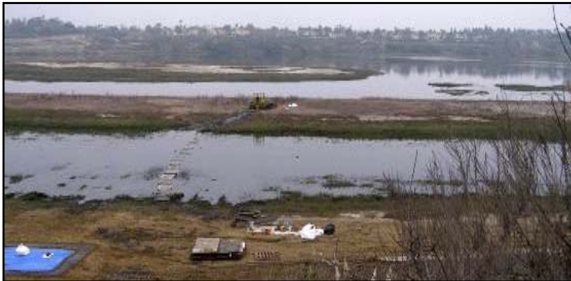
Construction Equipment and temporary bridge, Hotdog Island, Photo by Keane Biological, 15 March 2007
