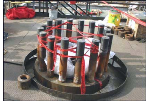
Access to the Valero reactor
