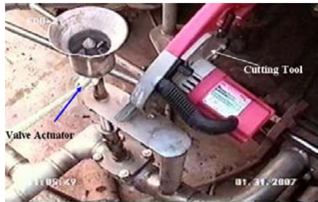
Exhibit 4-18: Diversion Box Valve Actuator & Cutting Tool.
