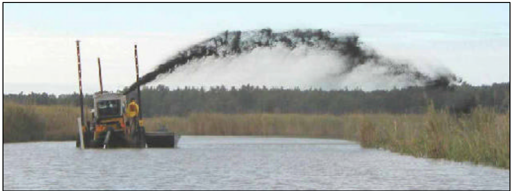
The Corps is spraying thin layers of dredged material to restore marshes as part of a demonstration project at Blackwater National Wildlife Refuge, Md. (USACE photo)
