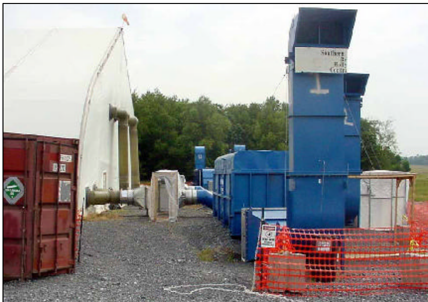
The containment structure air filtration system that is being used at Fort Detrick, Md. (Courtesy U.S. Army COE)
