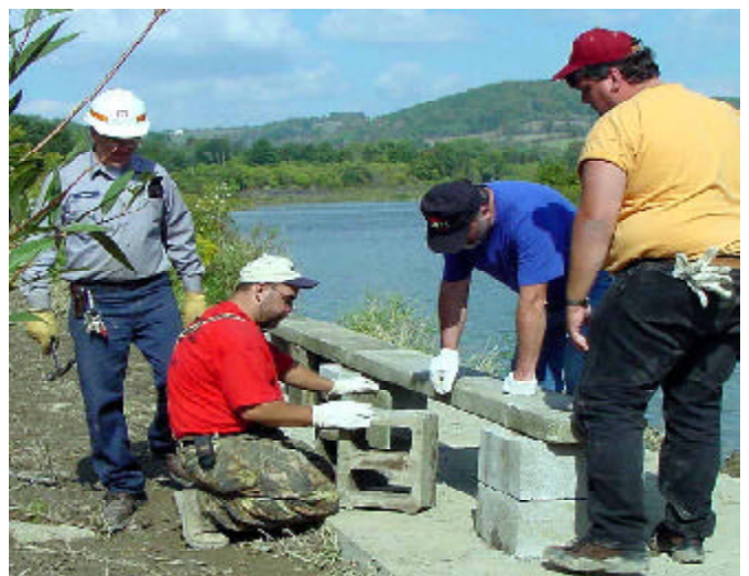
Dam operator Gary Miller (left) directs volunteers with construction of a handicapped fishing pier. (USACE photo)
