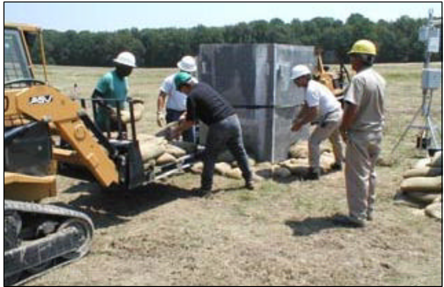
Workers at Lauderick Creek, Md., place sandbags around a barricade before detonating an unexploded munition. U.S. Army photo
