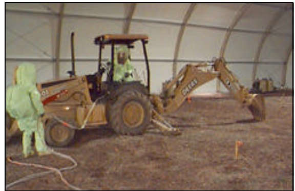
Wearing level A protection, workers excavate a medical waste pit at area B-11, Fort Detrick, Md. U.S. Army photo
