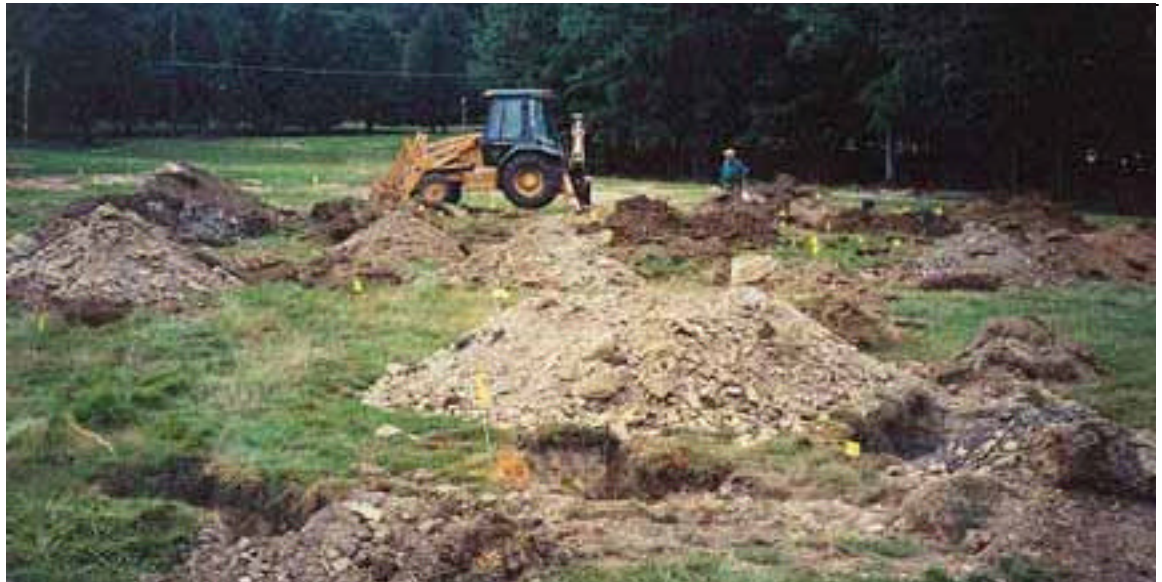
Workers excavate ground looking for unexploded ordnance. The individual anomaly sites, marked with flags, were identified by sophisticated metal detectors. (Photos courtesy U.S. Army)
