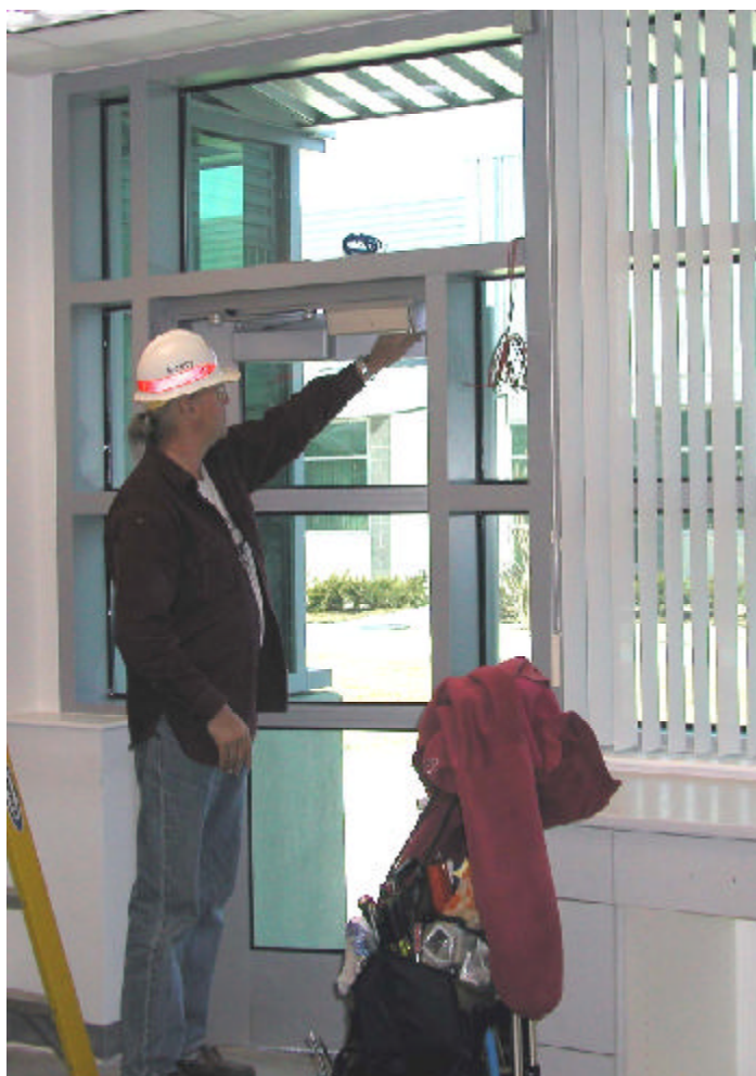
Woody Snyder inspects the installation of the security system at the Special Testing Laboratory.
