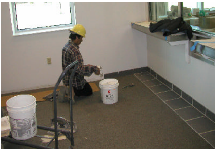
A worker installs baseboard tile at the front lobby of the Special Testing Laboratory.
