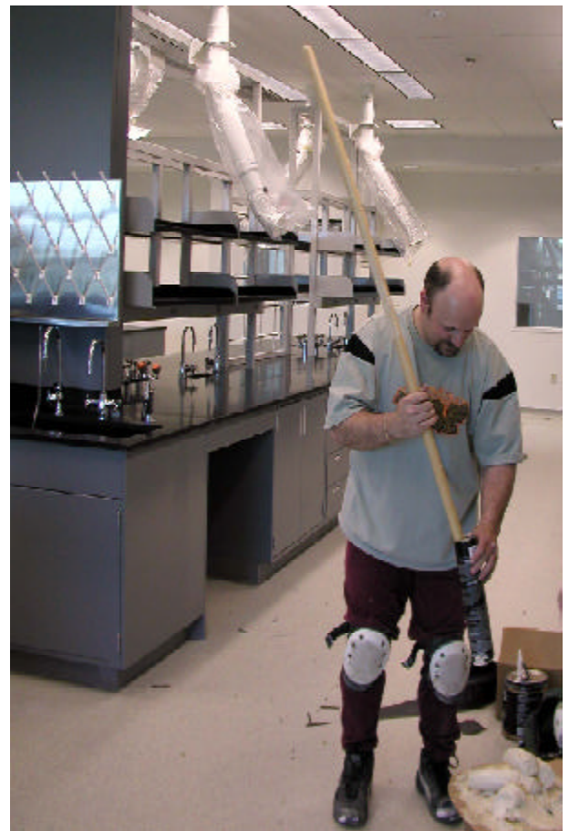
A worker retrieves the remaining caulk from a tube as part of the final detail work at the lab.
