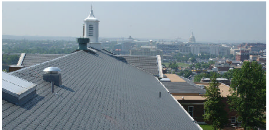
The roof was replaced with artificial slate. Though more expensive than asphalt shingles, it was one-third the price of real slate, while providing a 50-year life and restoring the original appearance.
