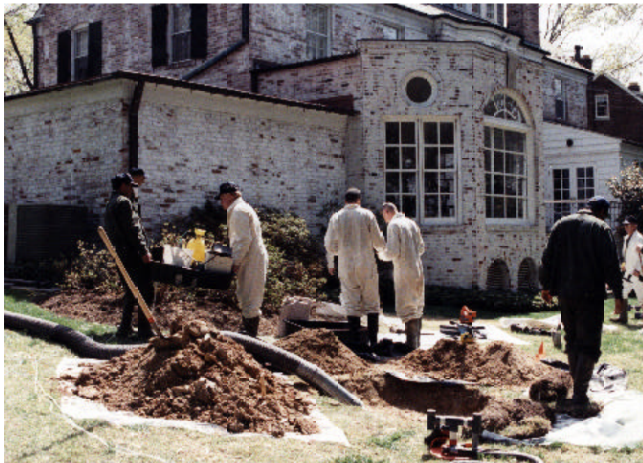
Workers search for buried munitions at a Spring Valley home. This area in Washington, D.C., has been the focus of a 10-year cleanup effort by Baltimore District. (Photo by Tex Jobe)
