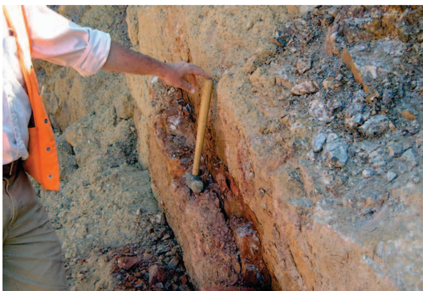
Figure 31. North-striking fault with red clay gouge developed in massive vuggy silica rock in the Superior quarry.
