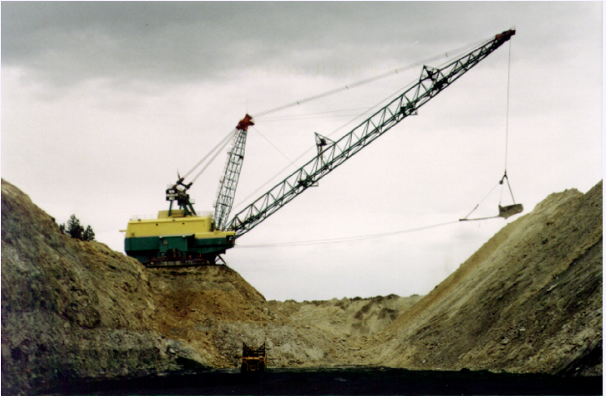
Figure MO-23. The operator's "touch"—note that the bucket is extended past the end of the boom. This Bucyrus-Erie 1570 dragline is sitting on the highwall and "spoiling" or dumping overburden on the low wall side of the pit.
