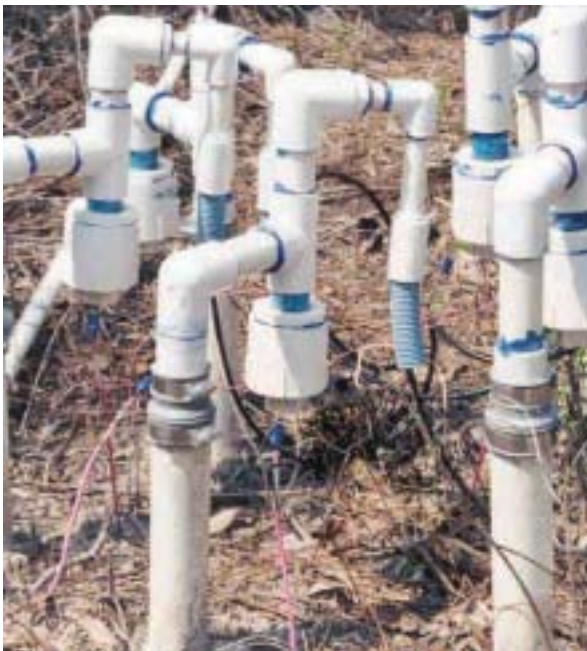
Figure 4. Proper installation of the right kinds of monitoring devices is important to obtain approval of changes and additions to the hydric soil indicators.
