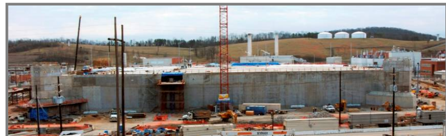
(upper) Work on the new HEUMF is 75% complete, with operations expected to begin in 2010. (lower) Artist’s rendering of the UPF.
