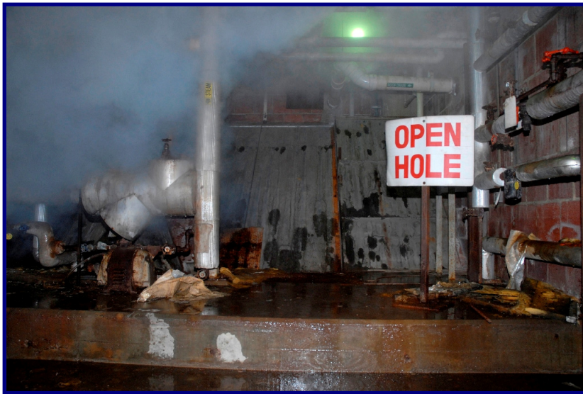
Fig. 13. Steam leaks indicative of deteriorating safety conditions in Building 9201-5.
