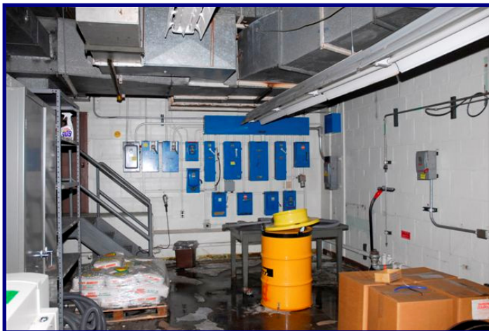
Fig. 14. Increasing safety concerns (note water on floor and numerous electrical panels) in Building 9204-4.
