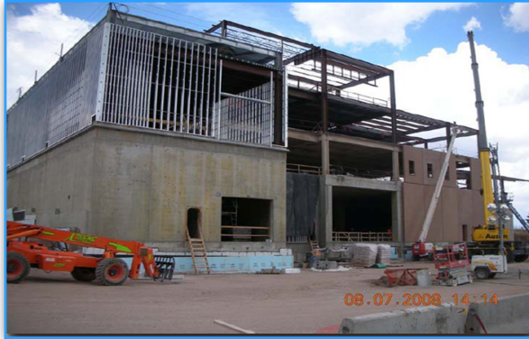
The completion of the CMRR project, currently under construction, will contribute to the Laboratory's nuclear facility consolidation efforts.
