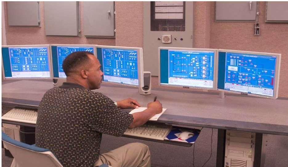
SAVANNAH RIVER'S TEF: Operator John Sanders tests the control systems at the nearly complete Tritium Extraction Facility (TEF) at the Savannah River Site in South Carolina. The facility is scheduled to begin operations in FY07. It's two main buildings are the Remote Handling Building and the Tritium Processing Building. Currently, all nine gloveboxes are installed and eight have been turned over for startup testing. TEF is part of NNSA's Tritium Readiness Program. There has been no new source of tritium in the U.S. since 1988.
