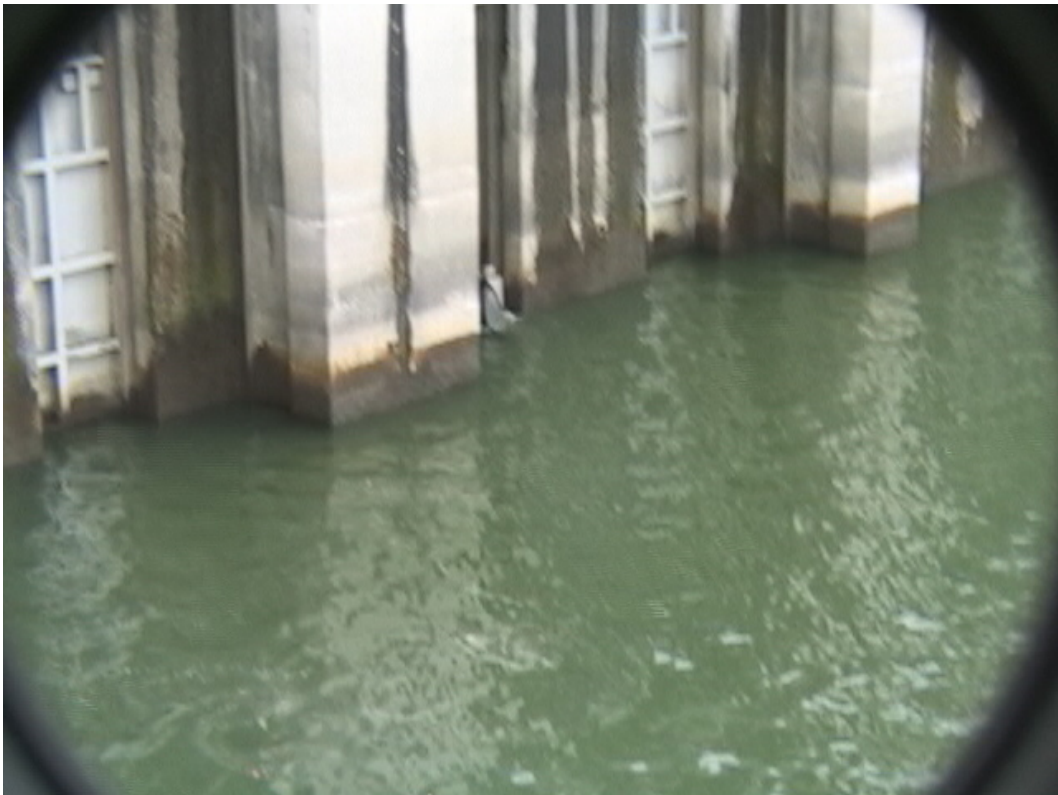
Poor quality still frame of C404 exiting over one of the floating orifice gates.
