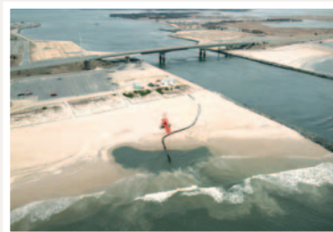
INDIAN RIVER INLET SAND BYPASS PLANT
